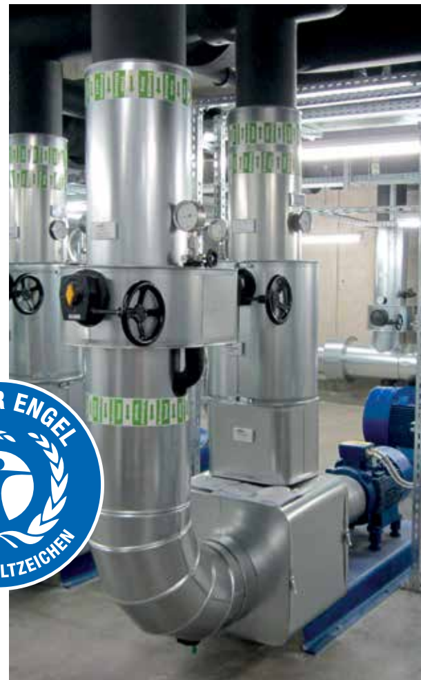
Heat generated by the Hawk supercomputer is used to heat the buildings, while the use of free cooling requires significantly less energy than traditional air conditioning systems
