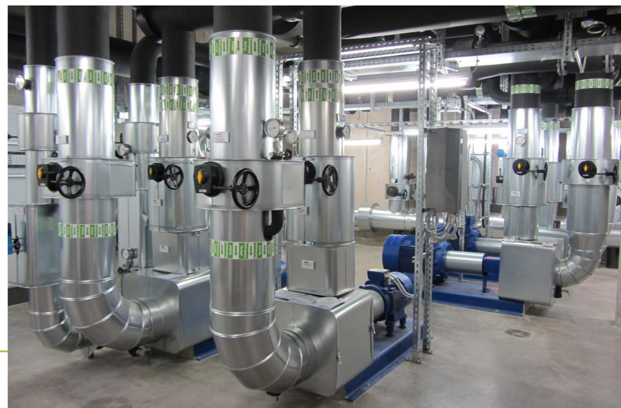
HLRS continues to investigate new opportunities to improve its energy efficiency, including in the operation of its cooling system.
