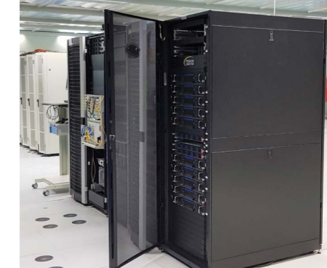
Installation of HLRS’s new system for COVID-related research.
