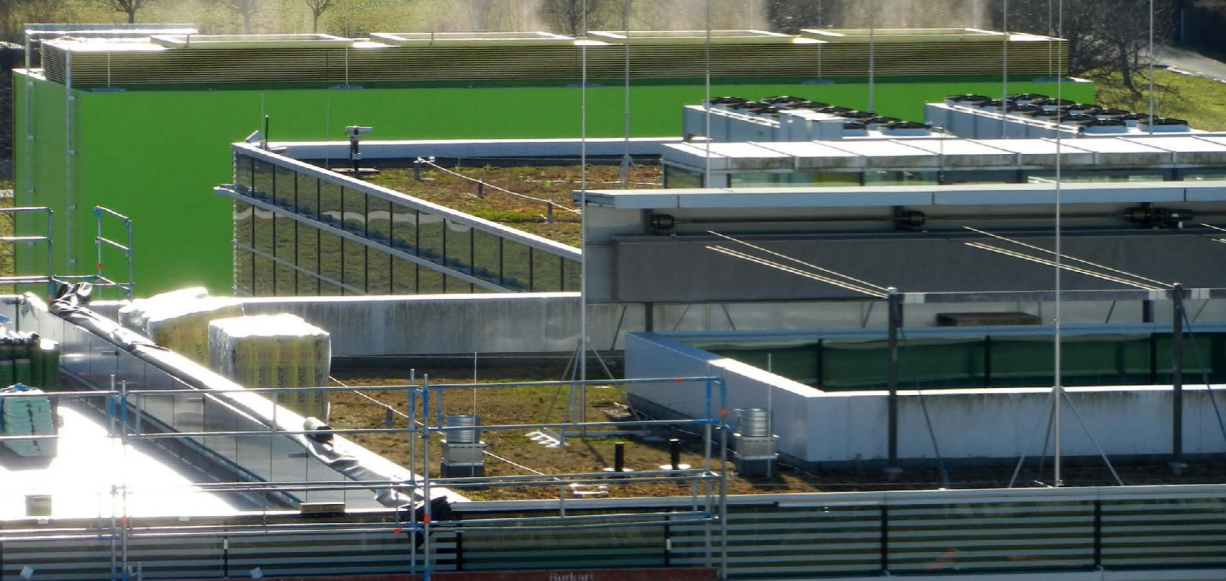
A dedicated cooling facility behind the HLRS main building keeps the center's computing systems from overheating.
